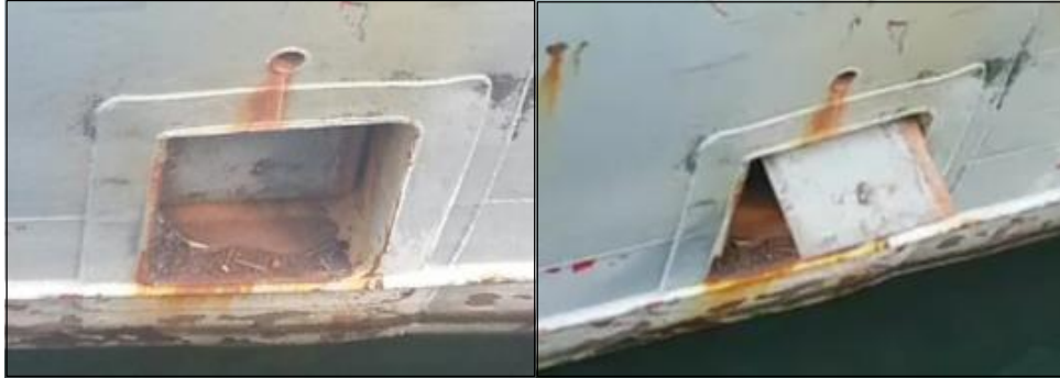
Fig. 2.7 Photo of discharge outfall on port stern side of F/V 501 Oryung.
