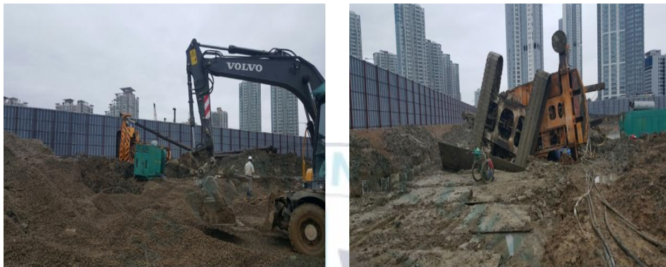
Fig. 3.4 Cheongna Central Complex evacuation accident of the Pile Driver[43]
