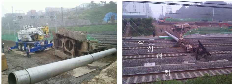
Fig. 3.1 Gyeongbu line evacuation accident of the Pile Driver[42]
