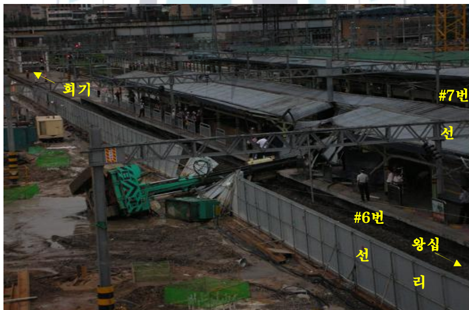
Fig. 3.2 Cheongnyangni line evacuation accident of the Pile Driver[42]
