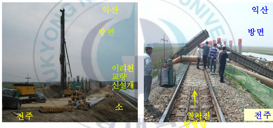
Fig. 3.3 Chuncheon Line evacuation accident of the Pile Driver[42]
