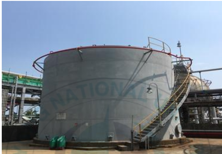
Figure 1. The Methanol Storage Tank
