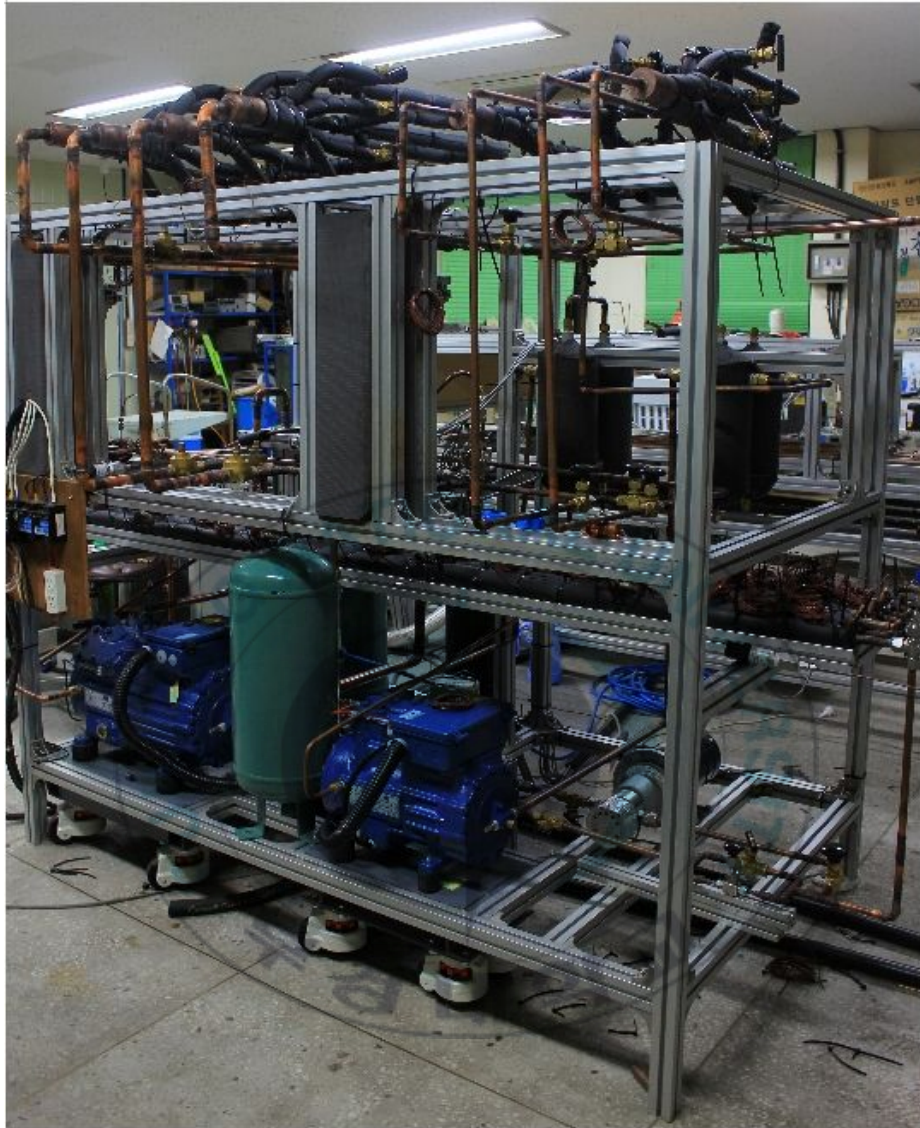
Pho. 2.1.1 Photo graph of CO 2 cascade refrigeration system
