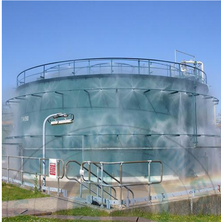
(a) Oil storage tank (8)
