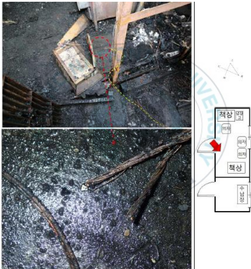
Photo 3. Melt marks generated from the power line in the direction of the electric heater.
