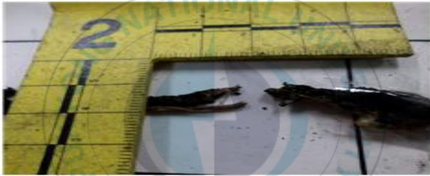
Photo 2. Separated wires of the wall-mounted fan found at the restaurant.
