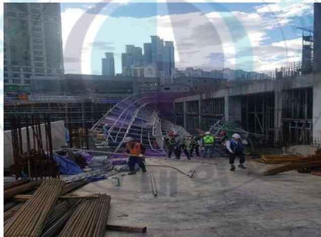
Fig. 3.4 Risk of falling due to the absence of wall joints
