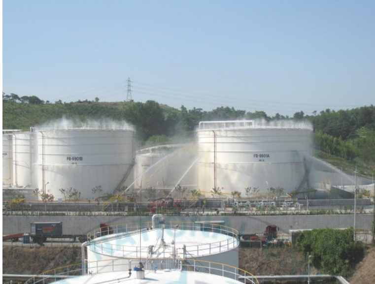
(a) Hazardous material storage tank
