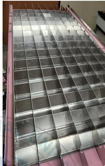
(b) Actual view of the air duct
