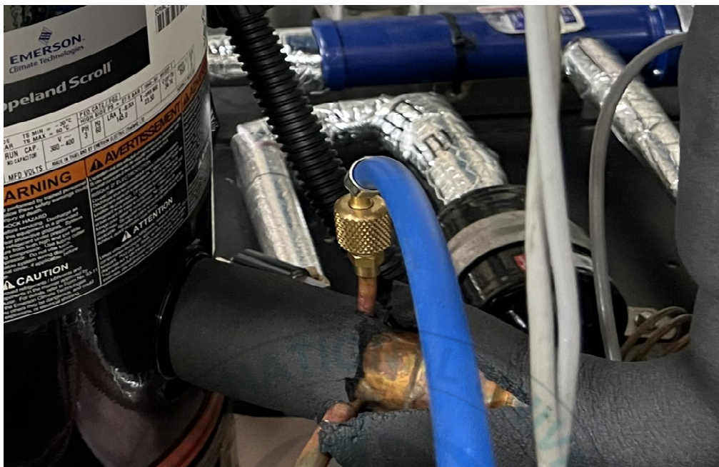
Fig. 3.4 Compressor suction side
