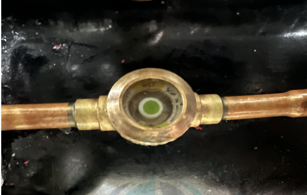
Fig. 4.19 Oil recovery pipe sight glass when the oil is adequate
