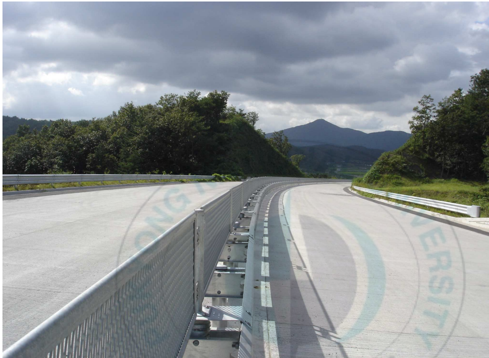
Figure 3.2 View of test field
