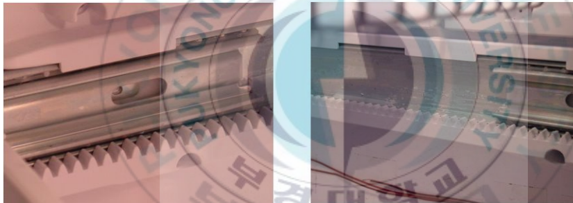
Fig. 28 The frost formation to the rail in the freezer
