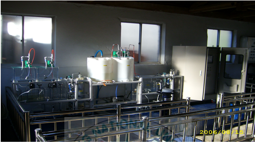
Fig. 3.6 Picture of pilot plant UF membrane filtration
