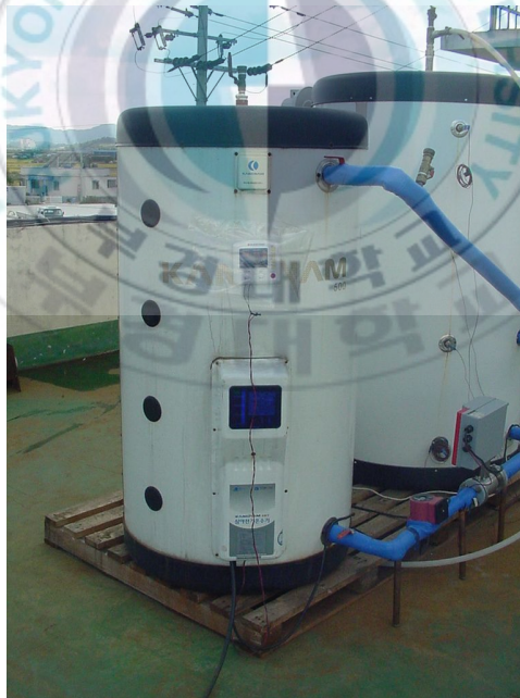
Fig. 6 Picture of the heating boiler
