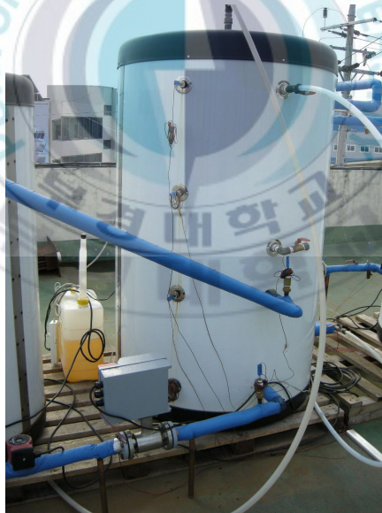
Fig. 9 Sensor point of storage tank
