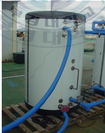
(b) Picture of the buffer tank
