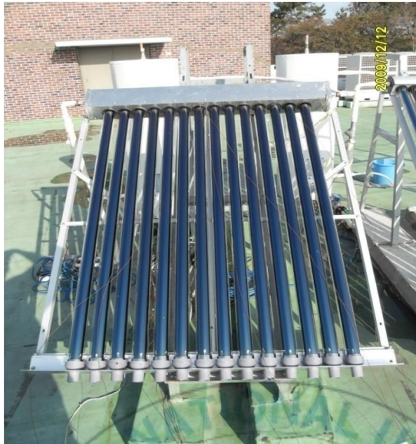
Photo. 1 Solar collector using PHP on the loop top
