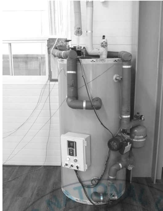
Photo. 3-2 View of a Storage tank
