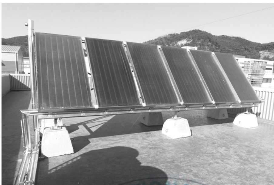
Photo. 3-1 View of solar collector
